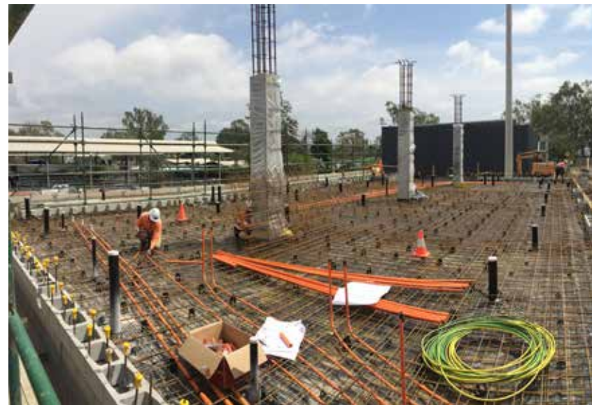
Construction of the new substation and chiller plant at UQ Gatton began during the year.
